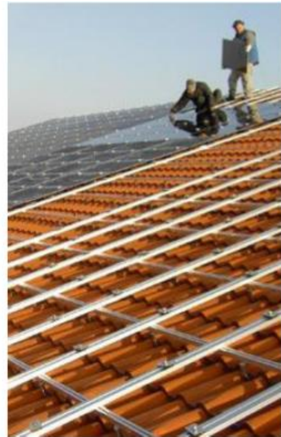
Installation in Spain
