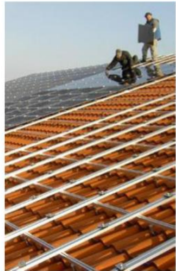
Installation in Spain
